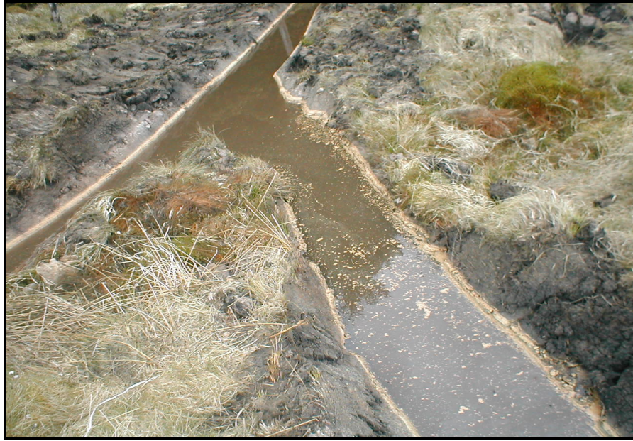
Figure 3. Drainage ditches flooded with water.
